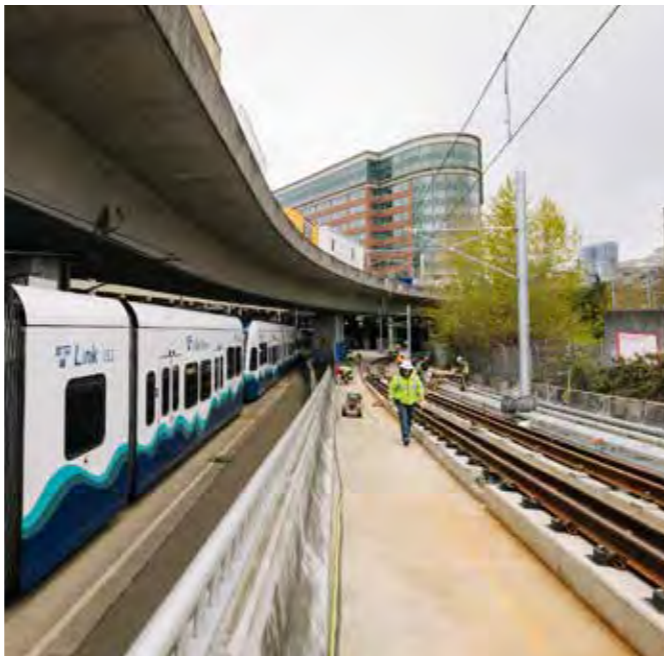
Connecting lines: tying the 1 and 2 lines together, East Link tie in completed.
