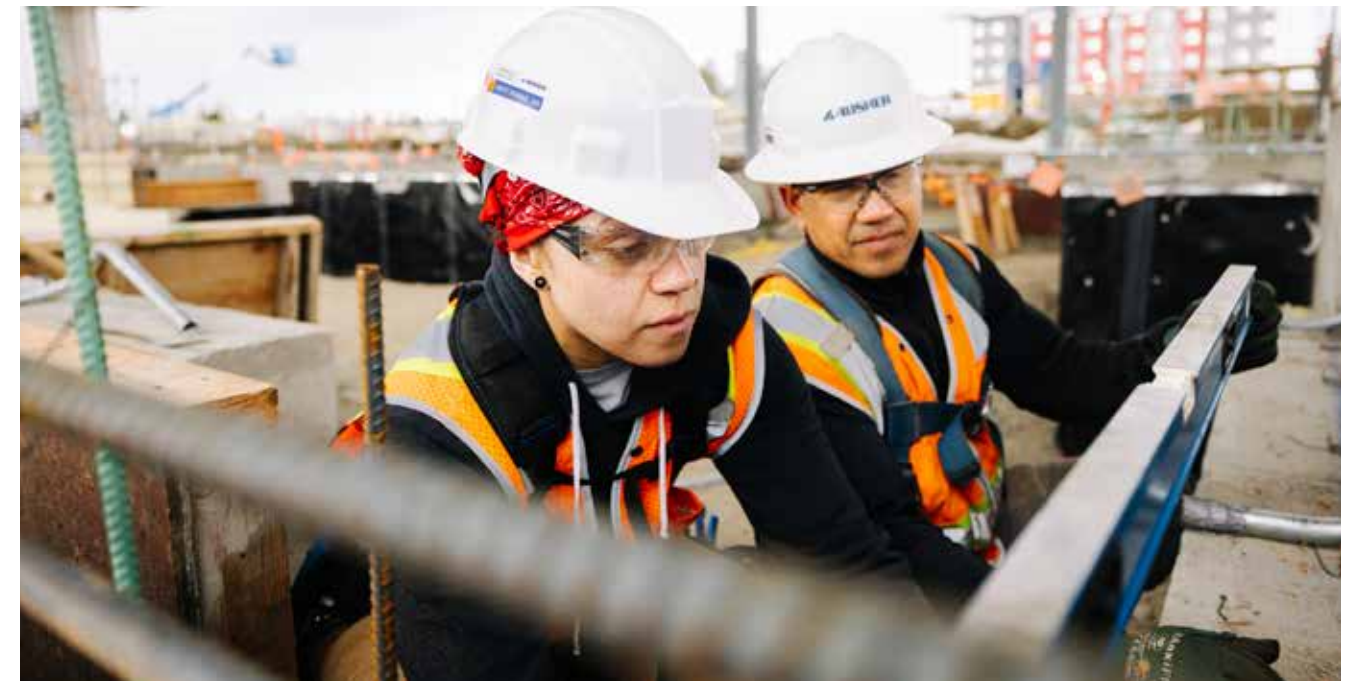
Construction workers check a level at the future Kent/Des Moines Link Station as part of the Federal Way Link Extension.
